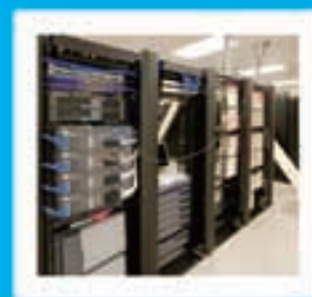
Monitoring the Data Center
